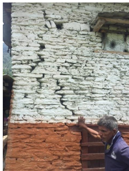
Tunnel blasting-induced house damage in Middle Modi HEP
